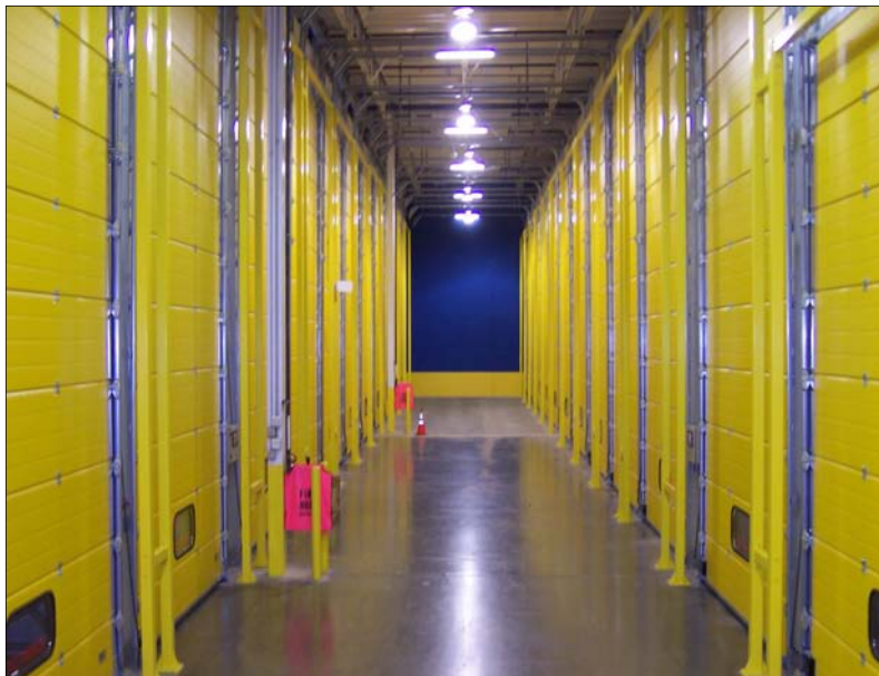
Fifty Room Ripening Facility, Coast Tropical, Los Angeles CA
