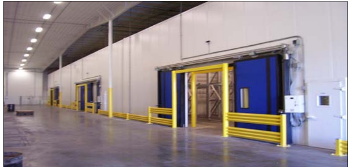
200 Pallet Ripening & Cooling Rooms with High Speed Doors
