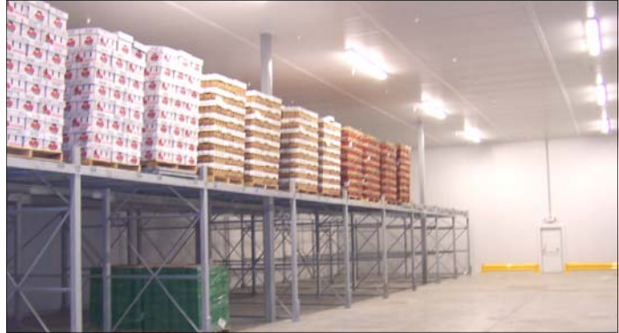
400 Pallet Storage Cooler For DiMare Fresh Tampa FL
