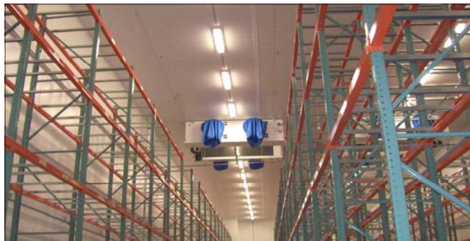
-10°F Freezer Room Whole Foods, Pompano Beach FL
